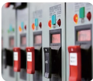
Power Control System
